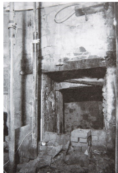
An old photo of work in the cellar of no. 12 Elvet Bridge. The door in the background opens into the old vannel, now a tunnel.
