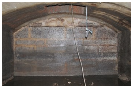
The entrance shaft, with the photographer's safety line and gas detector. Tidemarks and rusty stains can be seen on the walls.
